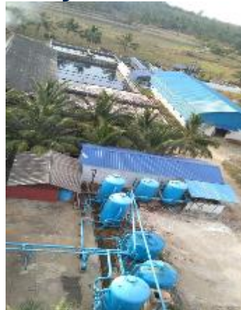
Effluent Treatment Plant recycles water
