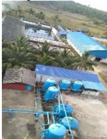
Effluent Treatment Plant recycles water
